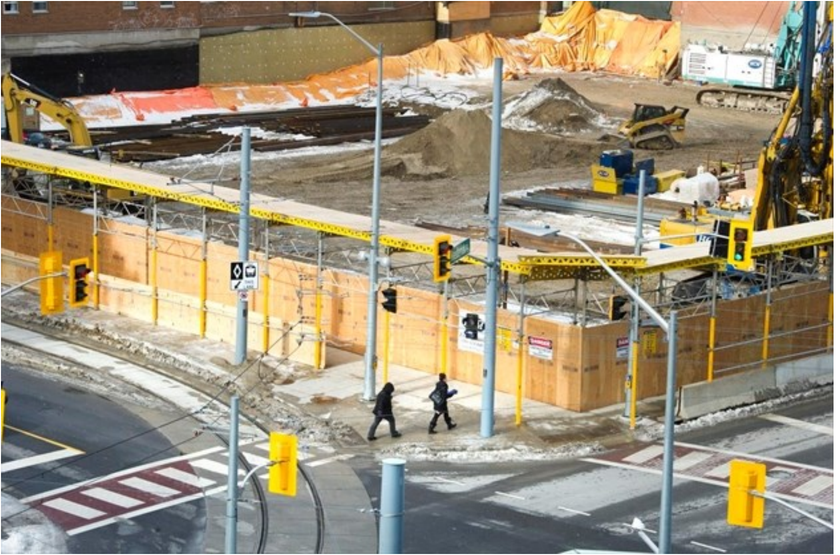
Construction continues on a building at Frederick and Duke streets. For its downtown development, Kitchener focused on the youngest group, the millennials, Luisa D'Amato writes. - Mathew McCarthy , Waterloo Region Record
